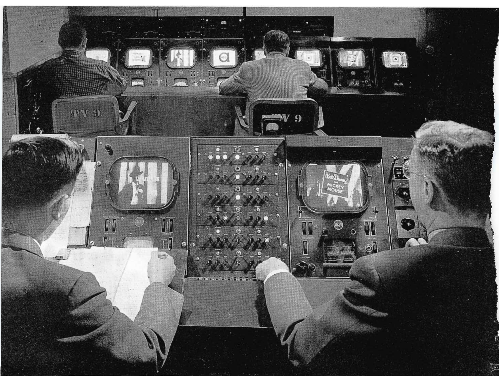
"FILM CENTRAL" for network operations. From this control room all the ABC film shows are fed to affiliates.
