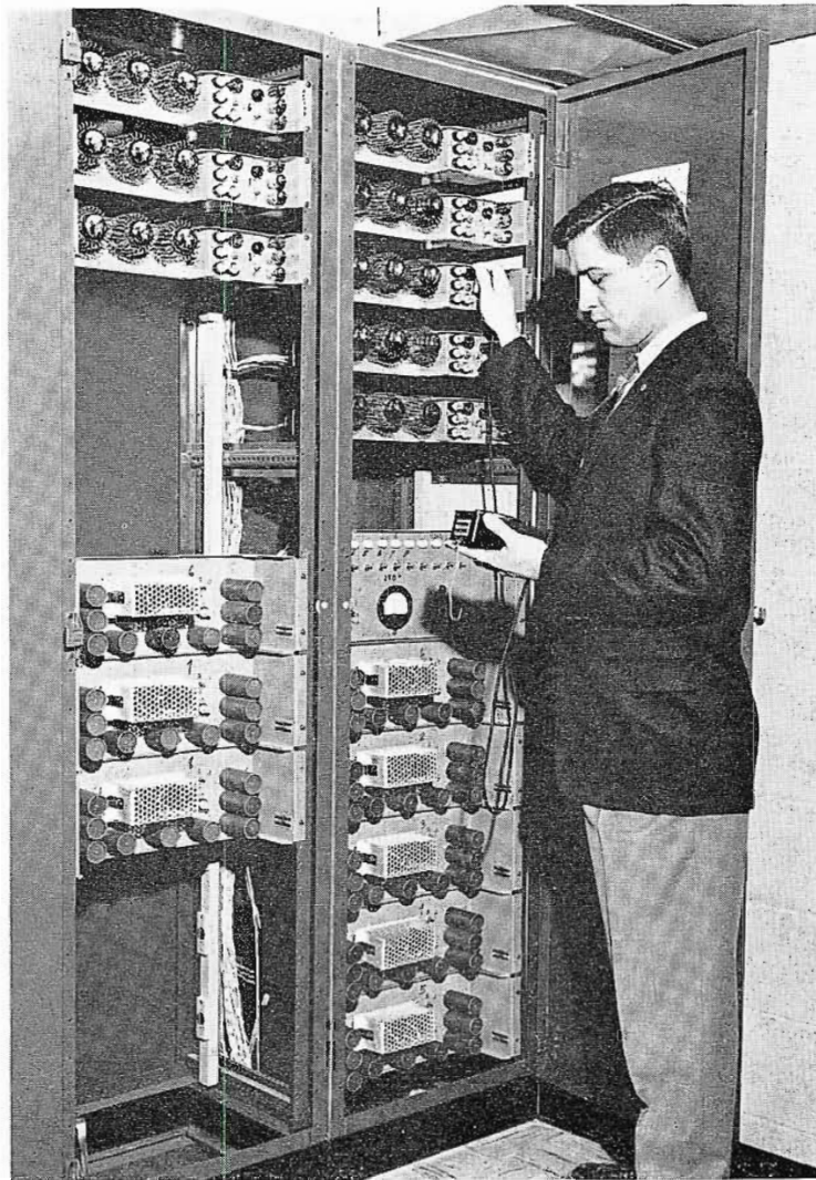
FIG. 17. Chief Engineer Jack Petrik at two racks which house power supplies for all 280-volt d-c requirements.
