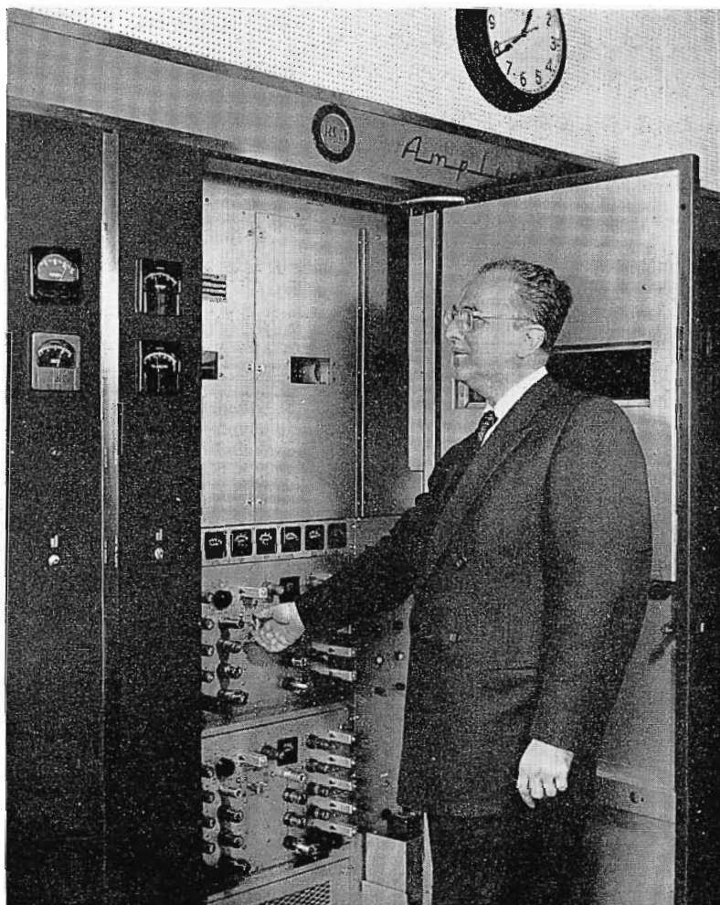
FIG. 1. Paul Von Kunits, WINS Chief Engineer, is shown making the one daily adjustment, the carrier level control, on the BTA-50G exciter modulator unit.
